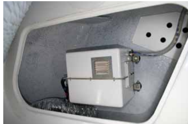
12,000btu Split system
